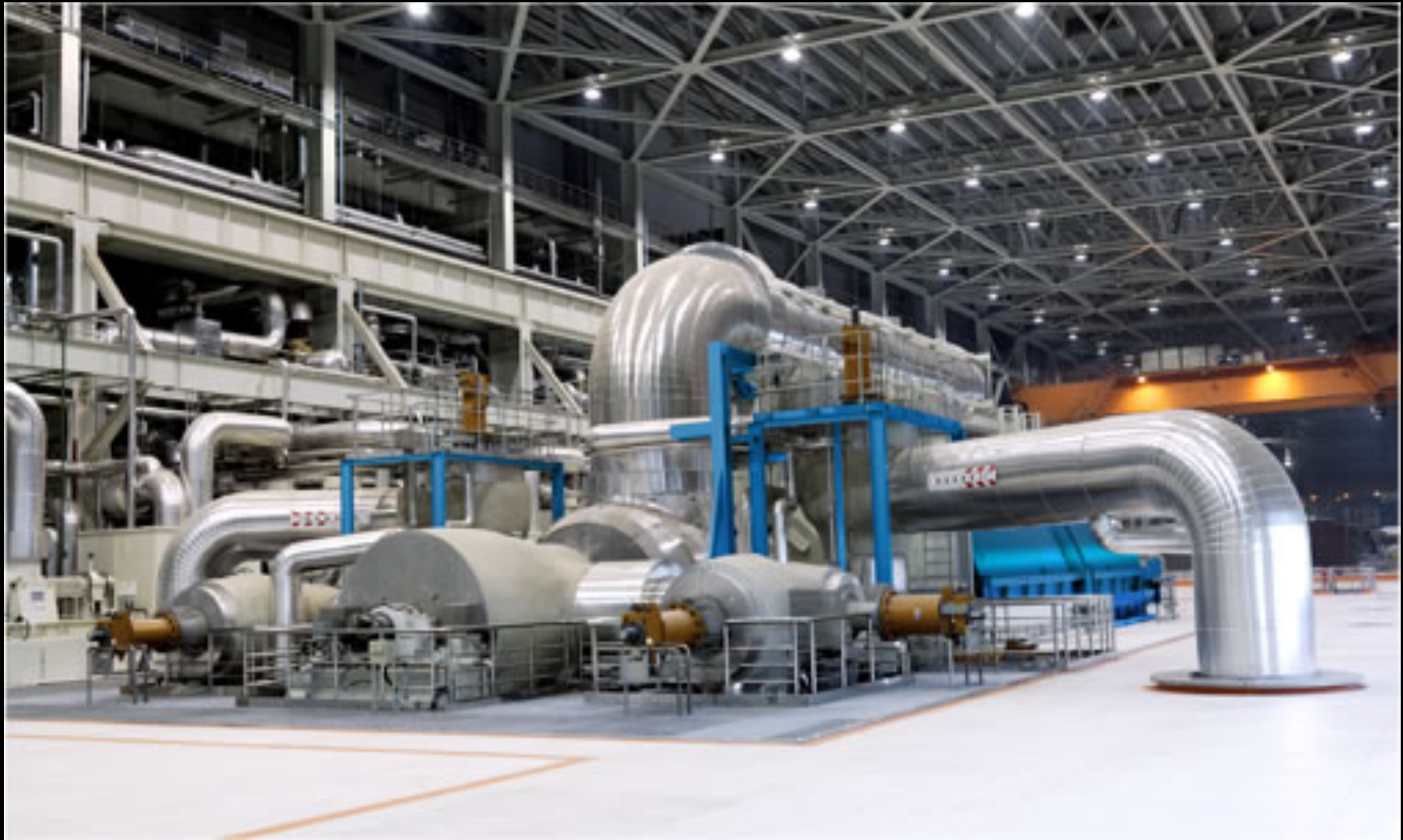
USC 1000MW unit at Shanghai Waigaoqiao III Power Plan
