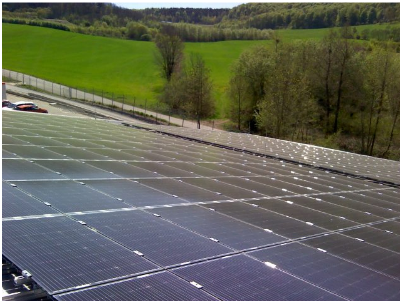
Photovoltaikdach, eigenes Werk Ute Bergner
